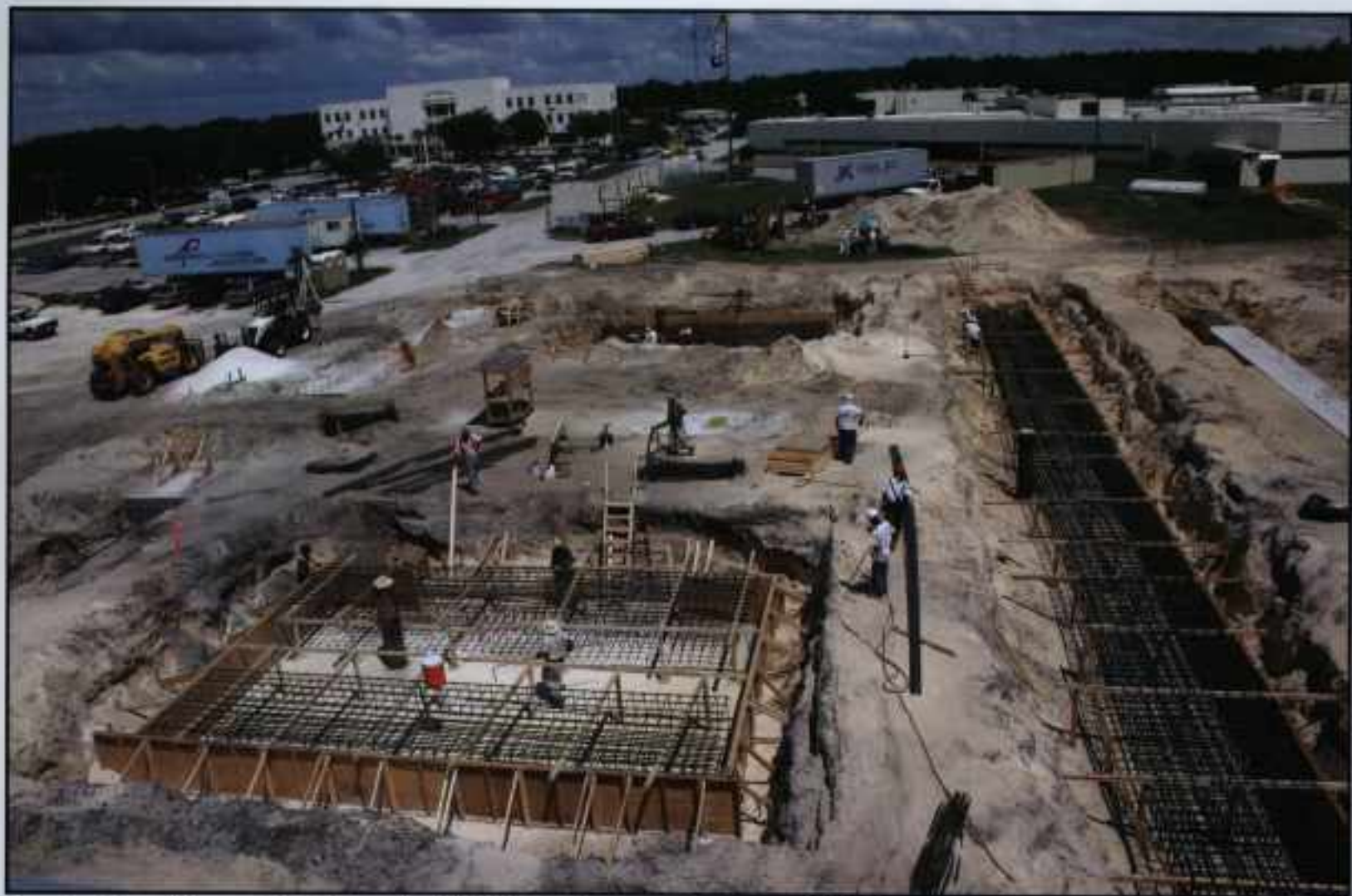
Construction of the new West Pasco Judicial Center began in the summer of 2004.
